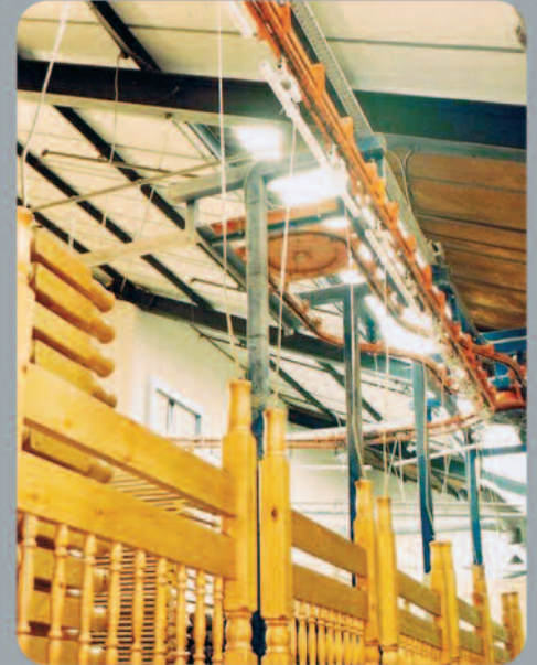
Accumulation of tall wooden parts prior to unloading, using power and free conveyor.
