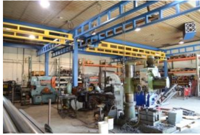
Free Standing Workstation Bridge Crane
