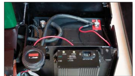
Power provided by two 12 volt, 70 amp hour batteries and onboard 110 volt charger
