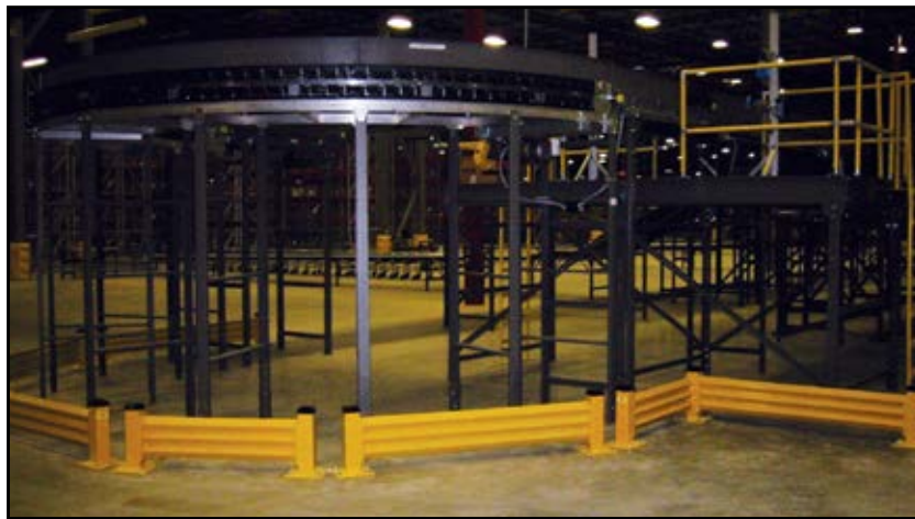
Guarding Overhead Conveyor
