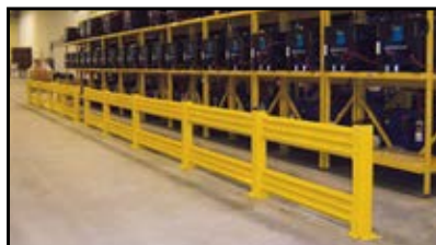
Guarding Battery Racks
