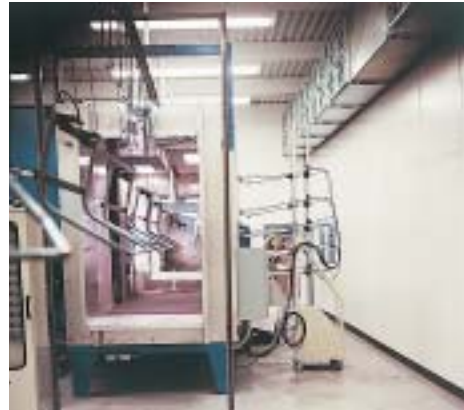
Powder coating application room.
